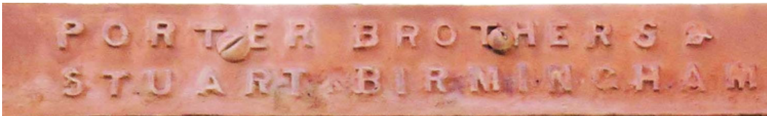
The Fitzroy Depot building, Porter Brothers & Stuart brand on a window head: Miles Lewis.
