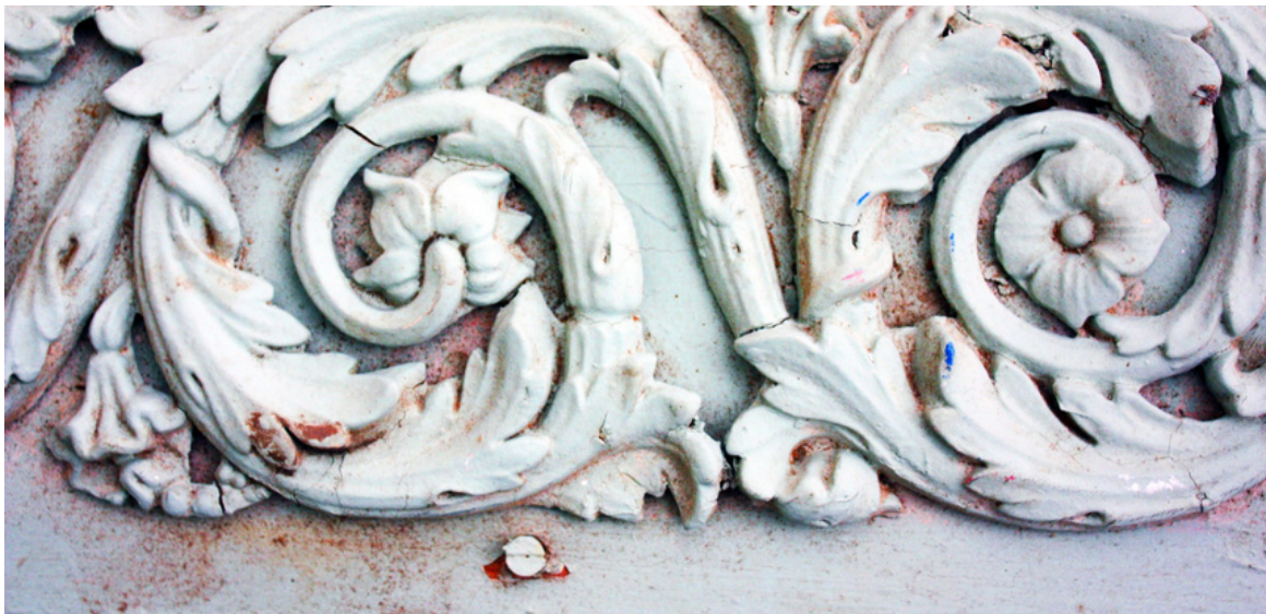
Wingecarribee, detail of papier mâché rinceau mounted on a board: Miles Lewis
