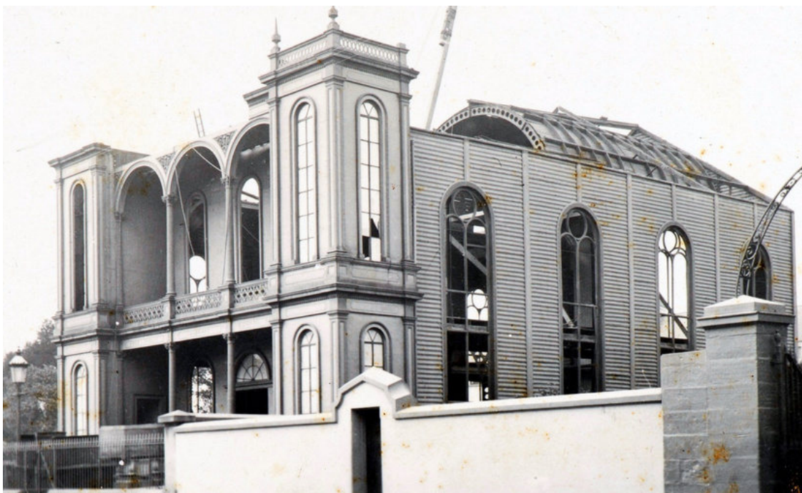
Former Free Presbyterian Church, Macquarie Street, Sydney, during dismantling, 1899: State Library of New South Wales PXE 1077 [cropped].
