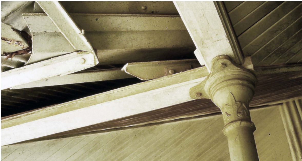
Detail at the corners of the verandah roof: Brian Kidd, Miles Lewis.
