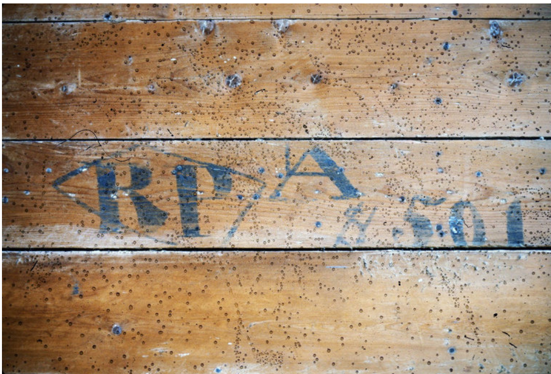
Iron house, 399 Coventry Street, 'RP' [Robert Patterson] monogram and lading marks, from the internal lining boards. Miles Lewis.
