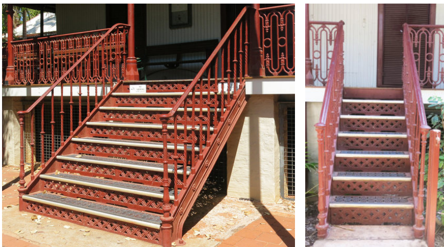
The main stair and the former south-west stair, now at the south-east: Miles Lewis.
