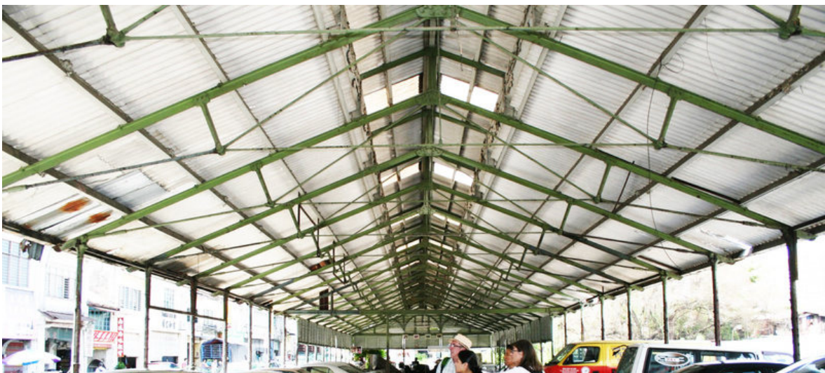
Market building roof, Georgetown Penang, by Andrew Handyside & Co of Derby, undated,: Peter Romey.
