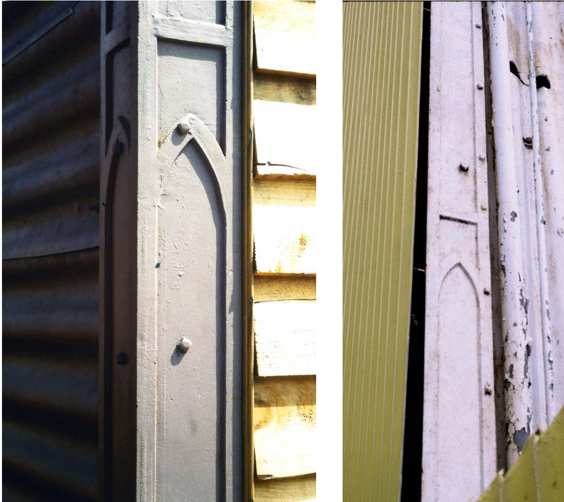
Store, rear 51 McKillop Street, Geelong, detail of corner column. Brown Brothers store, Ginn & Mercer Streets, Geelong, detail of column at rear corner (partly concealed by the modern yellow cladding at left: both Miles Lewis.
