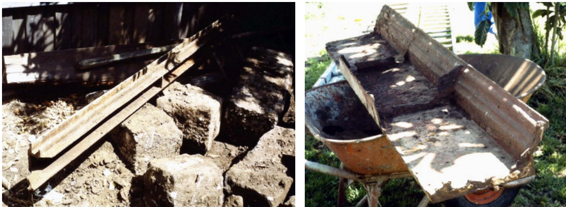
Corio Villa, a cast iron stanchion from the rear [corrugated iron] wall, and a cast iron gutter removed from the structure: Miles Lewis.
