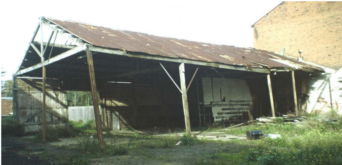
Store, rear of former Congregational Hall, 51 McKillop Street, Geelong, view prior to reconstruction. Photo, Miles Lewis.
