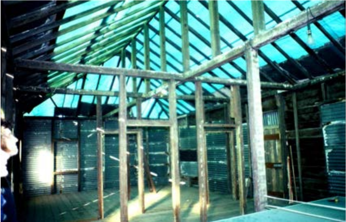
Former 1 Hoddle St, house frame as reassembled at Collingwood by Andrew Muir: Miles Lewis.
