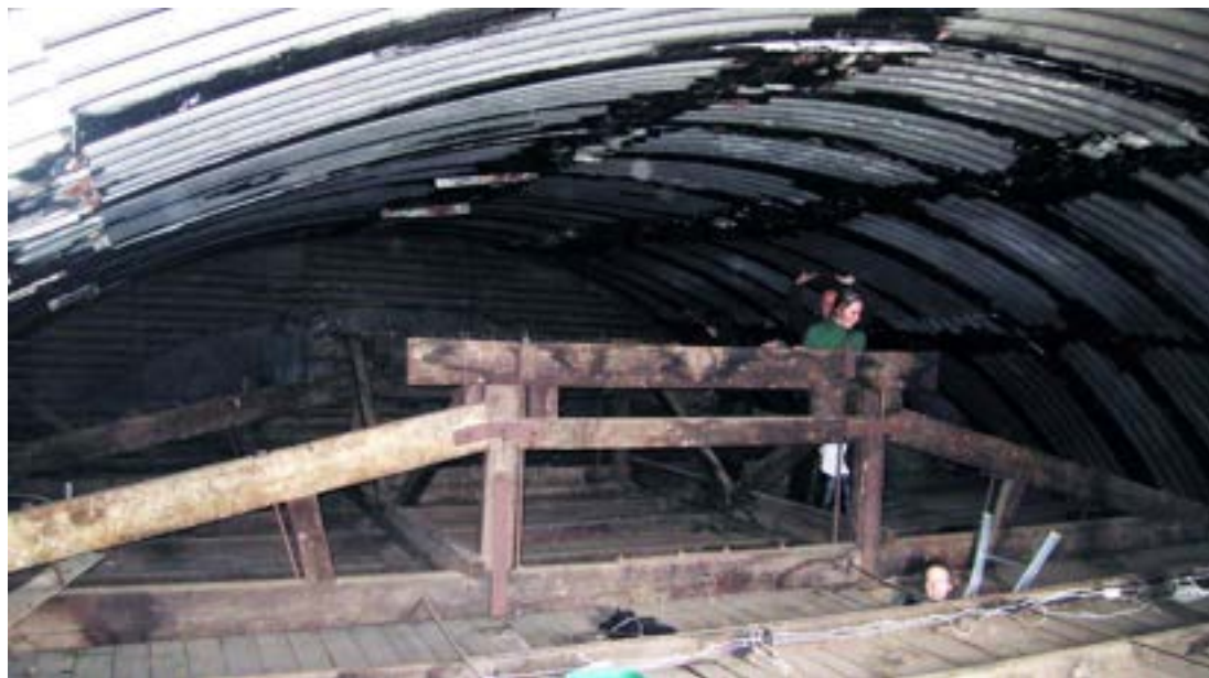
Brown Brothers store, roof space showing the queenpost truss suspension system: Miles Lewis.
