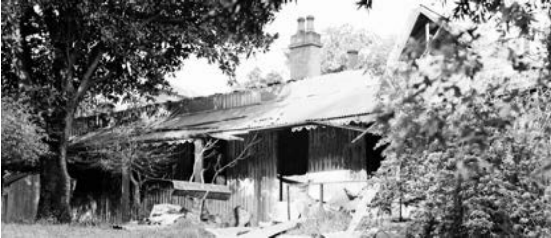
The Dingle, view during demolition, 1939, Alec Iverson, photographer: State Library of New South Wales ON 388/box 054/item 093 [cropped].
