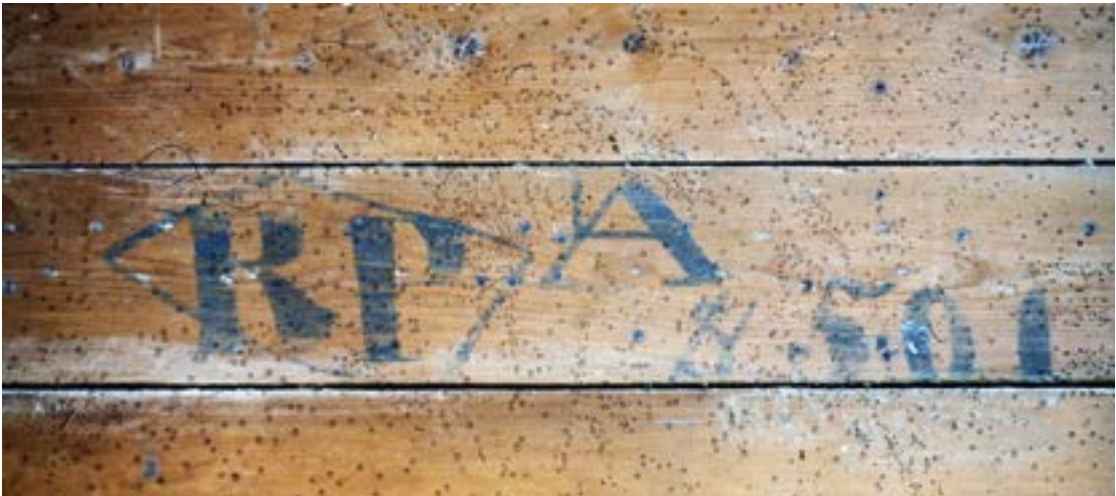
Iron house, 399 Coventry Street, 'RP' [Robert Patterson] monogram and lading marks, from the internal lining boards. Miles Lewis.
