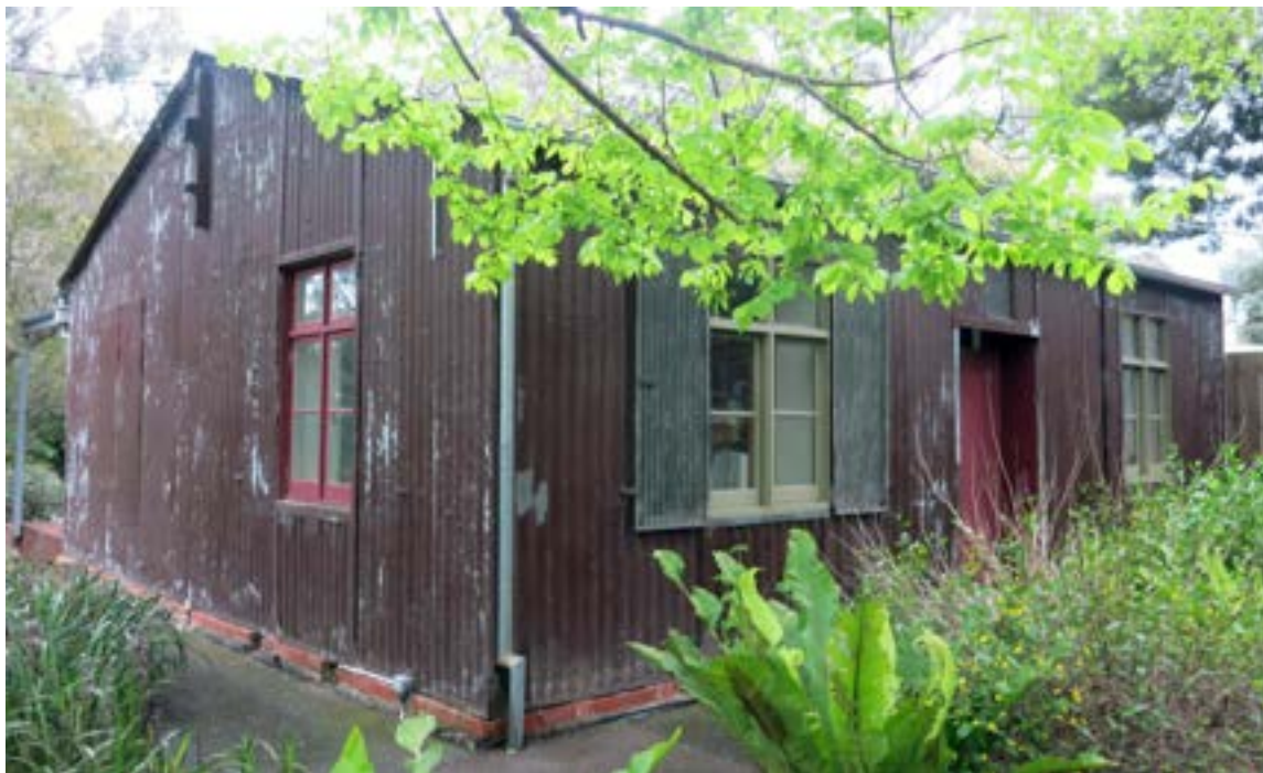
The ranger's huse, 161-168 Gatehouse St, Parkville by [Benjamin] Walmsley (or John Walker) fabricated c 1853, erected by 1862: Miles Lewis..
