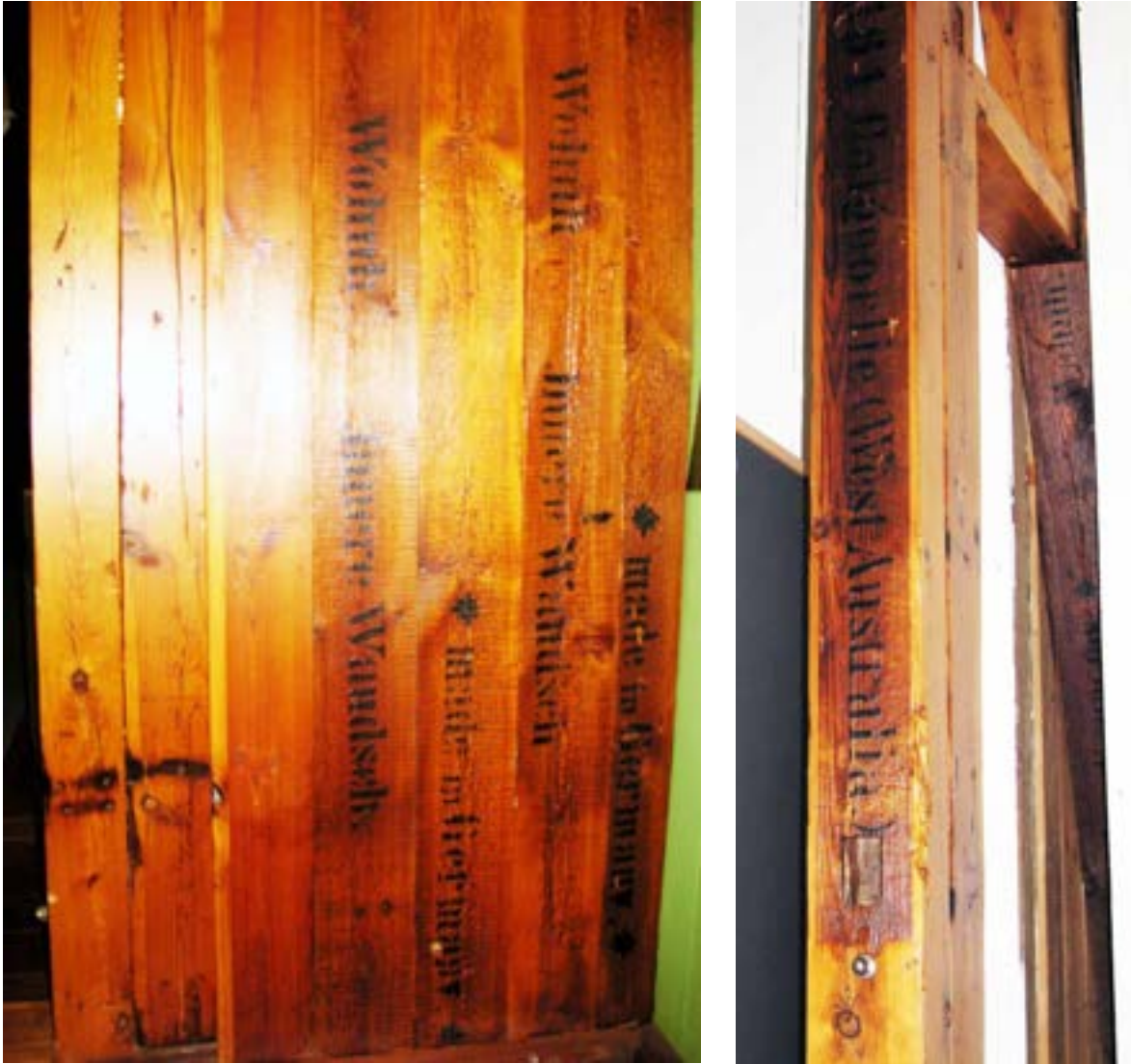
London and Hamburg Gold Recovery Company assay office, stencilled markings on the boarding and the posts: Miles Lewis
