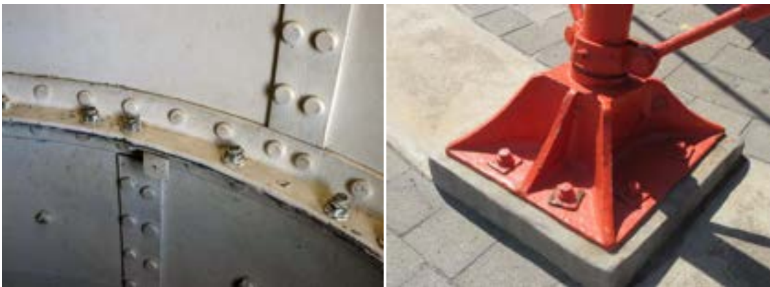
Iron lighthouse, Port Adelaide, interior detail; a base detail of the 1875 frame. Miles Lewis.
