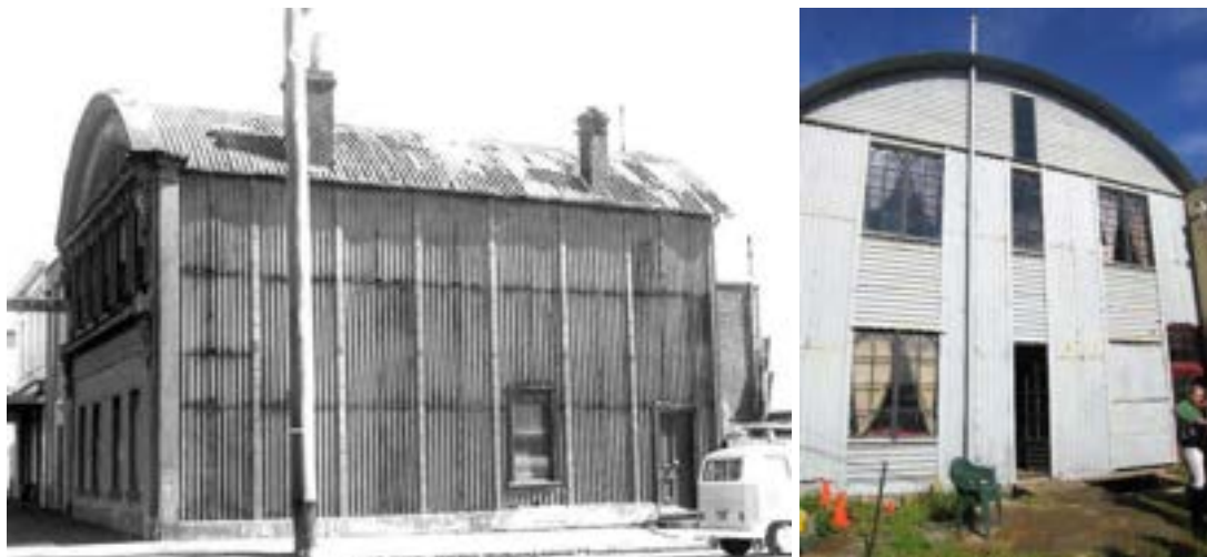
Brown Brothers store, mid-twentieth century side view; Peter Alsop. Rear view: Miles Lewis
