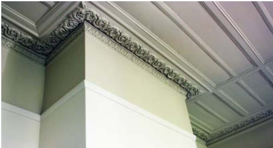
Wingecarribbee, a panelled ceiling with papier mâché border and cornice mould: Miles Lewis.
