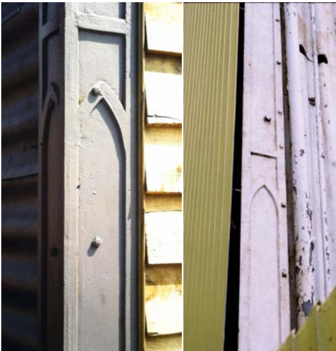
Store, rear 51 McKillop Street, Geelong, detail of corner column. Brown Brothers store, Ginn & Mercer Streets, Geelong, detail of column at rear corner (partly concealed by the modern yellow cladding at left: both Miles Lewis.
