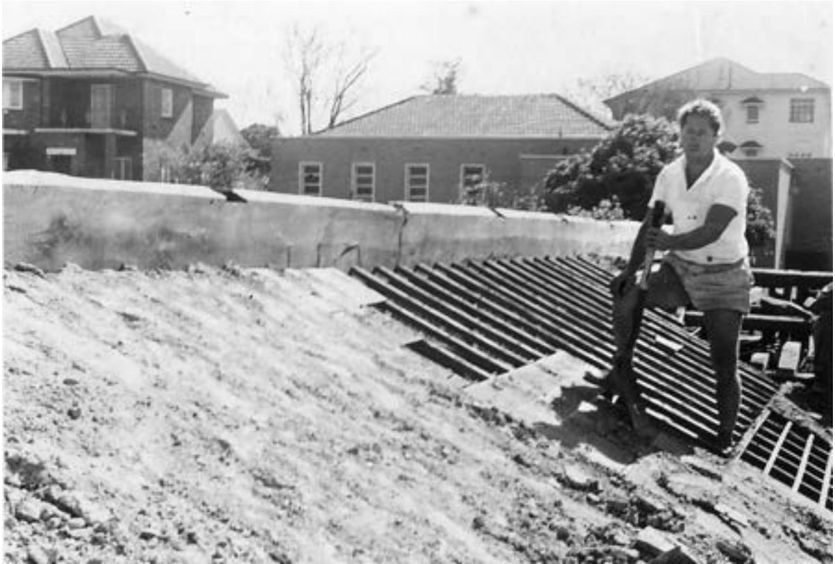
Dismantling of the verandah roof at the Brisbane site in 1962, showing the construction of round pole rafters, transverse boards, and mud, onto which the tiles were laid: Markwell collection.
