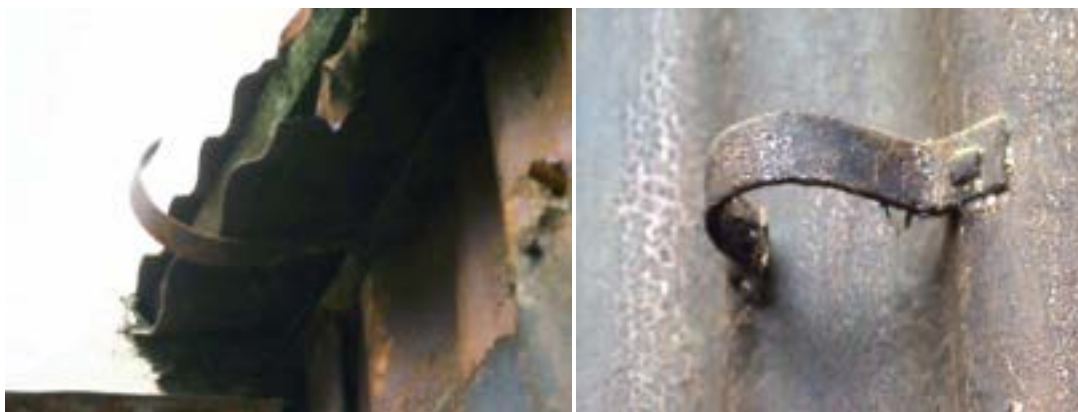
306 Bank Street, South Melbourne, gutter and downpipe brackets, believed to be original: Miles Lewis.
