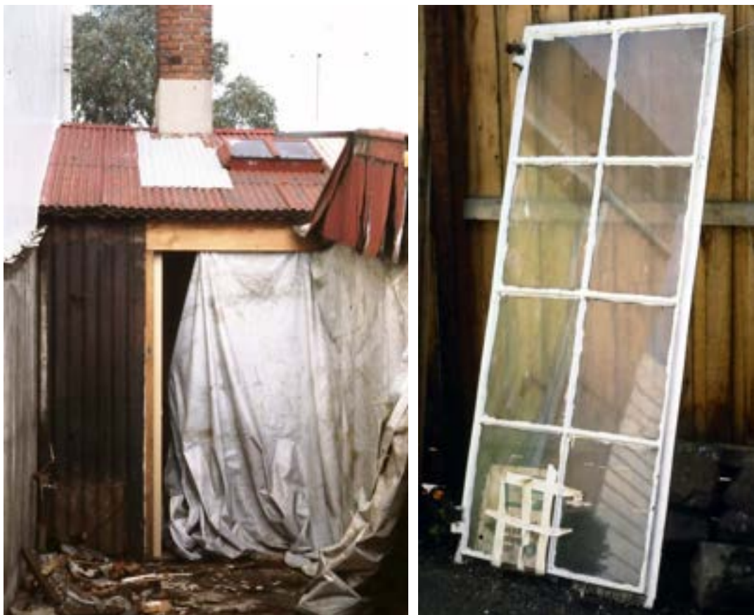
House at 306 Bank Street, South Melbourne, exposed rear wall as in 1983, and cast iron window sash: Miles Lewis.
