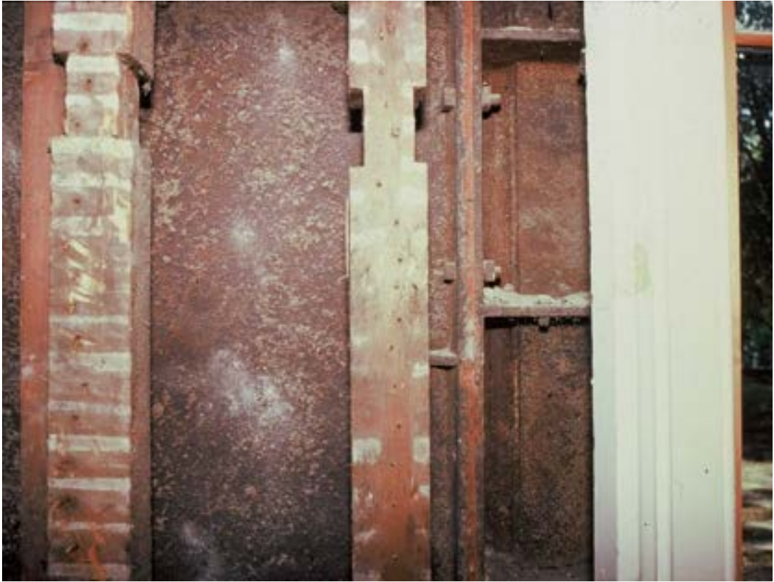
Corio Villa, Eastern Beach, Geelong, detail of the inside face of the west wall, showing timber studs stripped of lath and plaster, and behind these bolted iron tray construction. Miles Lewis.
